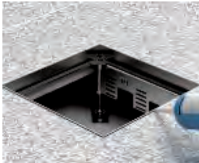
Laying the floor covering on the cassette frames Work the floor covering to the cassette frame. Seal the remaining gap between the floor covering and the cassette with suitable materials.
