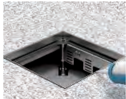
Laying the floor covering on the cassette frames Work the floor covering to the cassette frame. Seal the remaining gap between the floor covering and the cassette frame with suitable materials.
