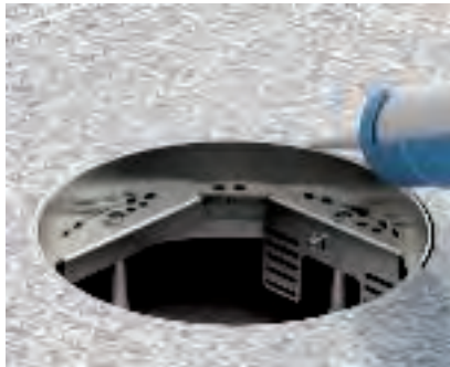
Laying the floor covering on the cassette frames Work the floor covering to the cassette frame. Seal the remaining gap between the floor covering and the cassette with suitable materials.
