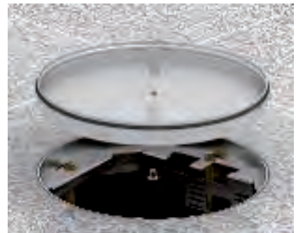
Mounting of a threaded sleeve This work step takes place before the floor covering is laid in the cassette. Drill a fastening hole for the threaded sleeve (Ø 8 mm). Insert the threaded sleeve and fasten it.
