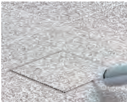
Laying the floor covering in the RKN cassette Lay the floor covering in the cassette and stick it down. Seal the remaining gap between the floor covering and the cassette with suitable materials.
