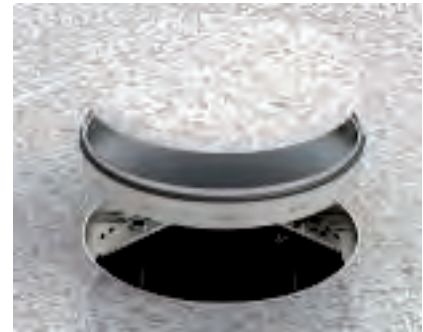
Laying the floor covering in the RKR cassette Lay the floor covering in the cassette and stick it down. Seal the remaining gap between the floor covering and the cassette with suitable materials.
